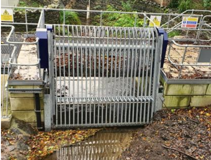
Automatic back-racking screen in Hazelwalls Park, East Staffordshire
