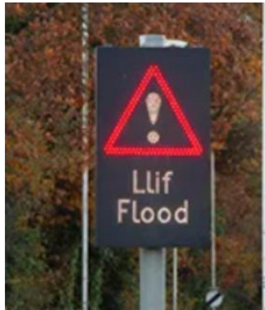
VMS flood warning signs in Edingale, Lichfield, (connected to level monitors) to advise of flooded roads
